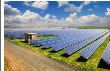
A solar farm
